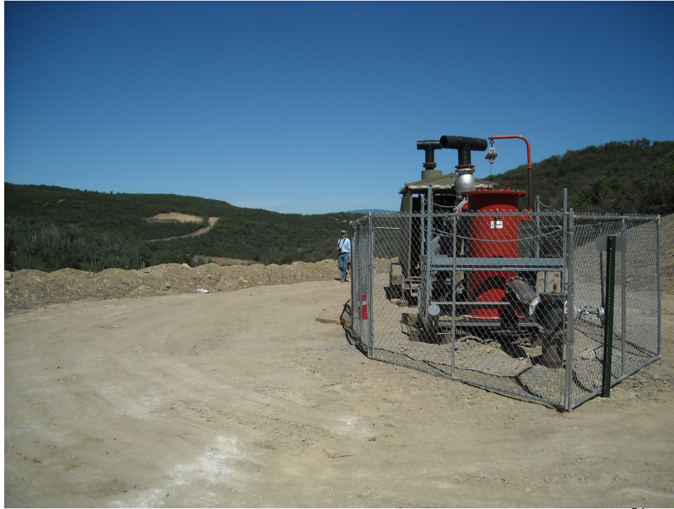
Methane Venting Above the West Elk Coal Mine in Colorado. 54
