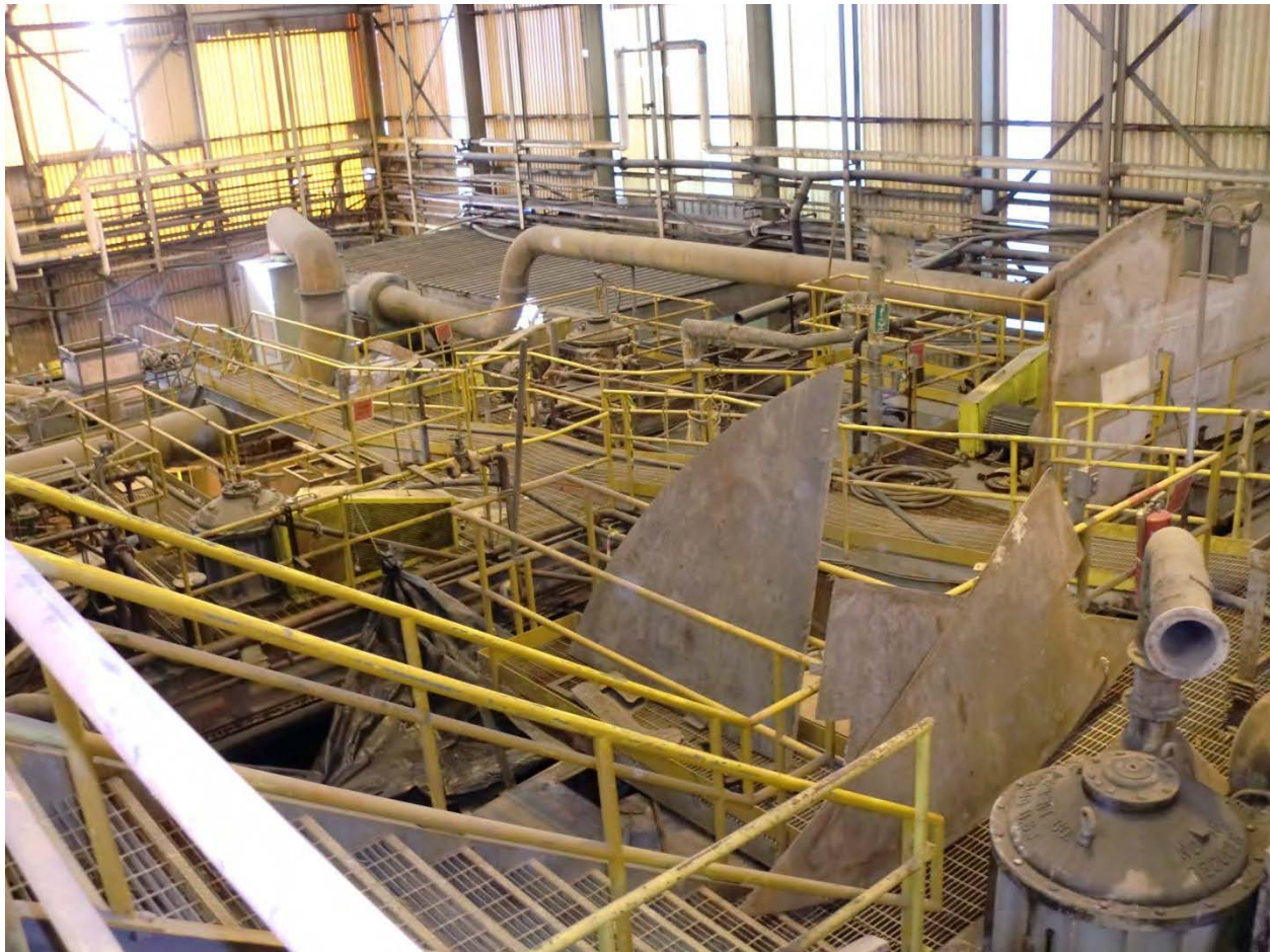
Photo 20. View inside the main solution leaching building. Walkways are over large leaching vessels and tanks. Photo taken by M. Linden, 10-27-11.
