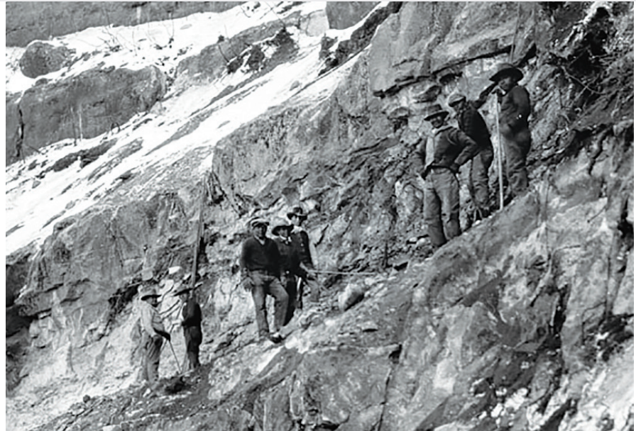
ABOVE: Havasupai trail crew working on upper Bright Angel Trail construction, Grand Canyon National Park, 1930. NATIONAL PARK SERVICE LEFT: Havasupai women gather near Red Butte to express opposition to Canyon uranium mine near Grand Canyon National Park. AMY S. MARTIN
