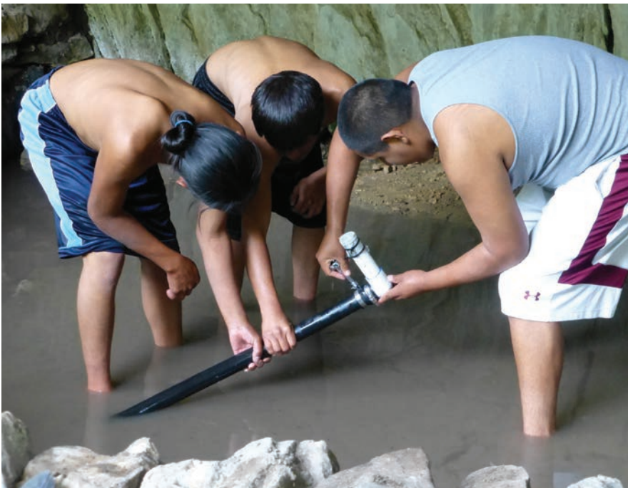
Hopi youth work on a drainpipe in the newly built water-catchment at Castle Springs.
